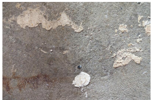
Adhesive contamination of concrete sub-floors
